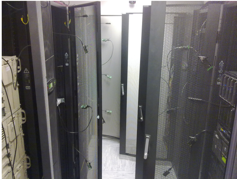
Figure 6.3: Picture of the network deployment at the datacenter.
